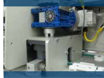
Variable Speed Drive
